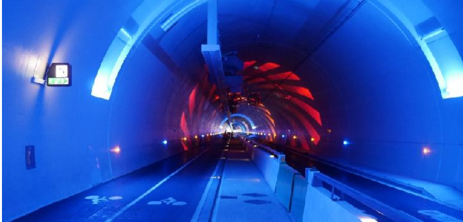
Figure 8 - Tunnel de la Croix-Rousse : Second tube dedicated to sustainable mode of transport.
